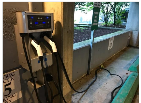
Marine Parking Garage EV Charging Station
